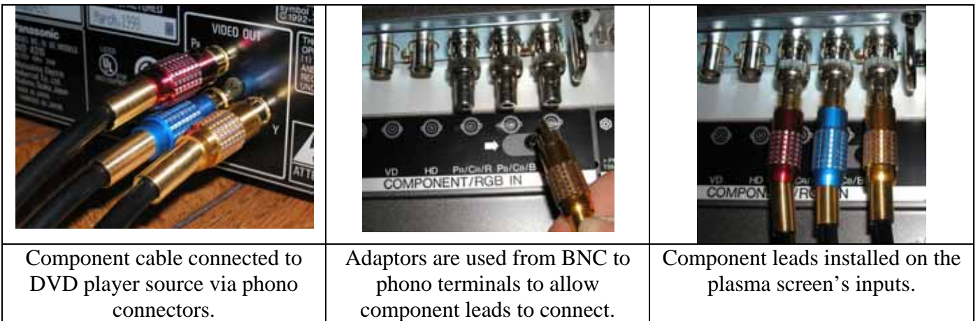
Figure 5. Connection of component video from DVD player to plasma screen, with the use of phono to BNC adaptors.
